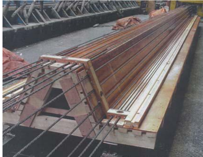
Figure 2.42. Prestressing strands and formwork used for production of SCFRC sheet piles (Walraven 2007)
