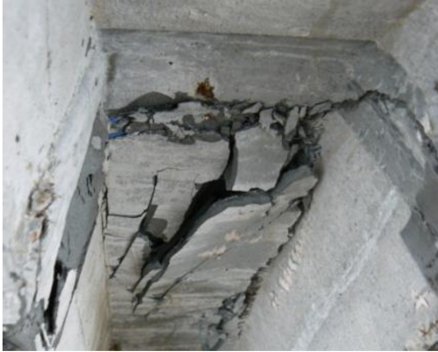
Figure 5.47. Damaged region of UHPC Pile 1 at the end of the lateral load test
