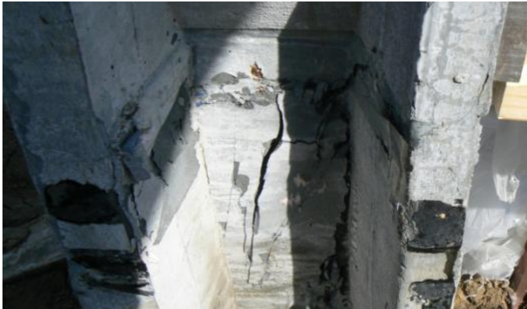
Figure 5.43. Initial shear cracking in web of UHPC pile P1 at a lateral load of 22.8 kip (101.3 kN)
