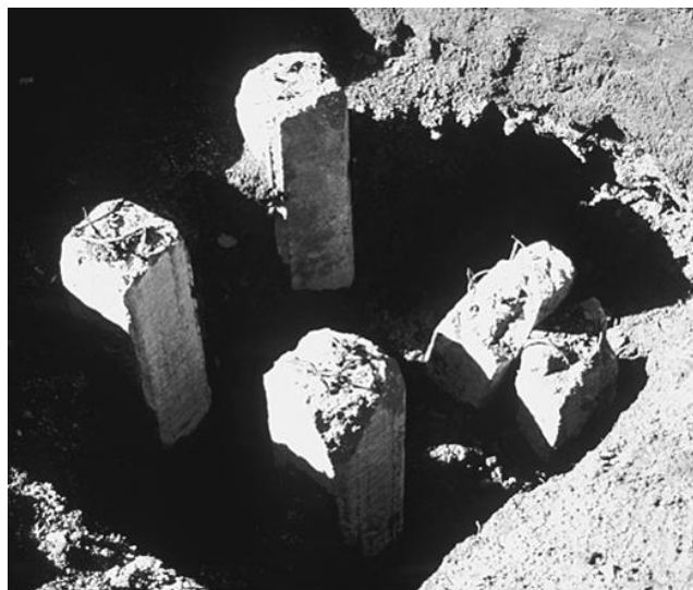
Figure 1.3. Damage to the tops of driven concrete piles due to unsuitable driving hammer size (Salgado 2006)
