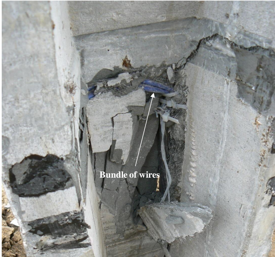
Figure 5.49. Shear failure region of UHPC pile P1 after the lateral load test with some cracked UHPC pieces removed
