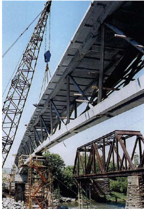
Figure 2.38. Placement of the second half segment of the Sherbrooke bridge on the falsework bent (Blais and Couture 1999)
