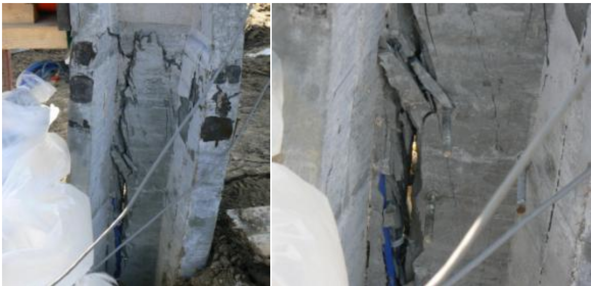
Figure 5.44. Views of the shear cracking on the east side of the web of UHPC pile P1
